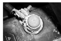
Corroded Cable Connection
