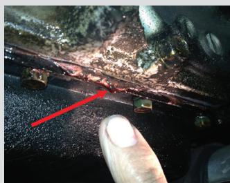
Leak due to gasket not conforming to pan irregularities
